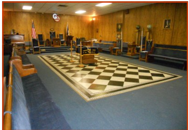
Brother Dean Jones has completed the newly tiled floor around the Altar.
